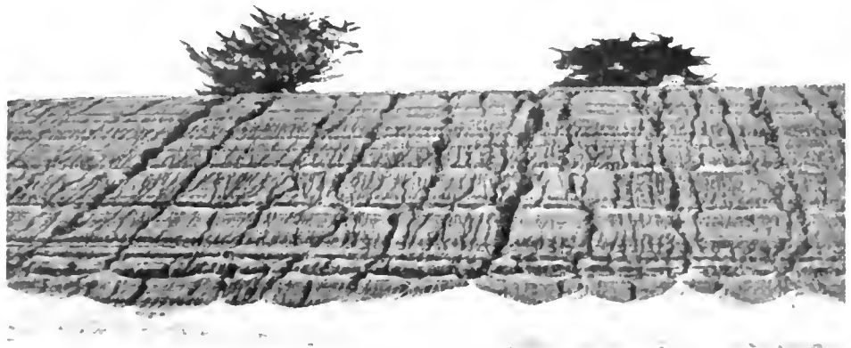
Untreated 2:1 slope after rain, showing result of erosion
